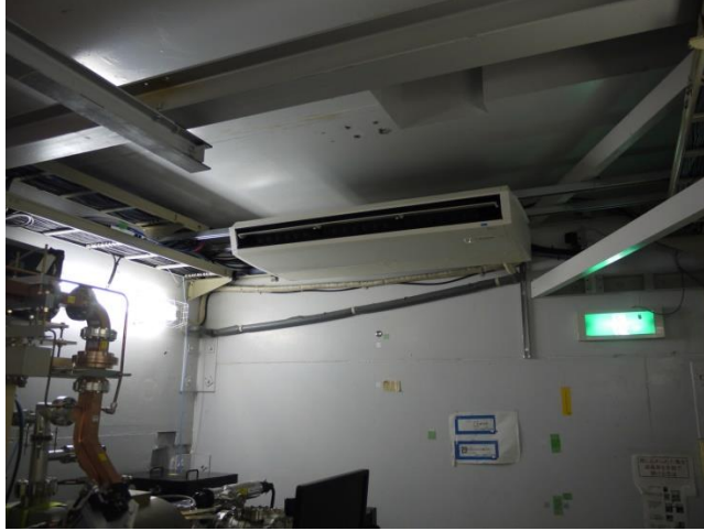
Figure 19: Mitsubishi Electric air conditioner
