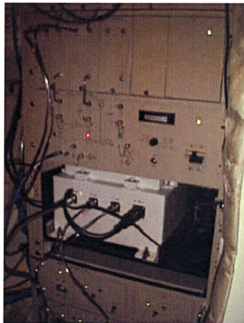
Figure 3.12. The front-end system in the center-hub of the 11m antenna. Upper: down converter and line equalizer, lower: local oscillator and phase calibrator unit
