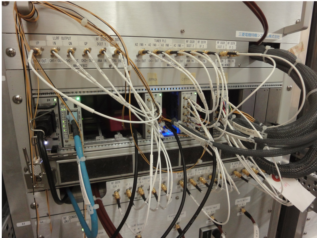
FIGURE 2.9: microTCA-based LLRF controller installed in Super KEKB.
