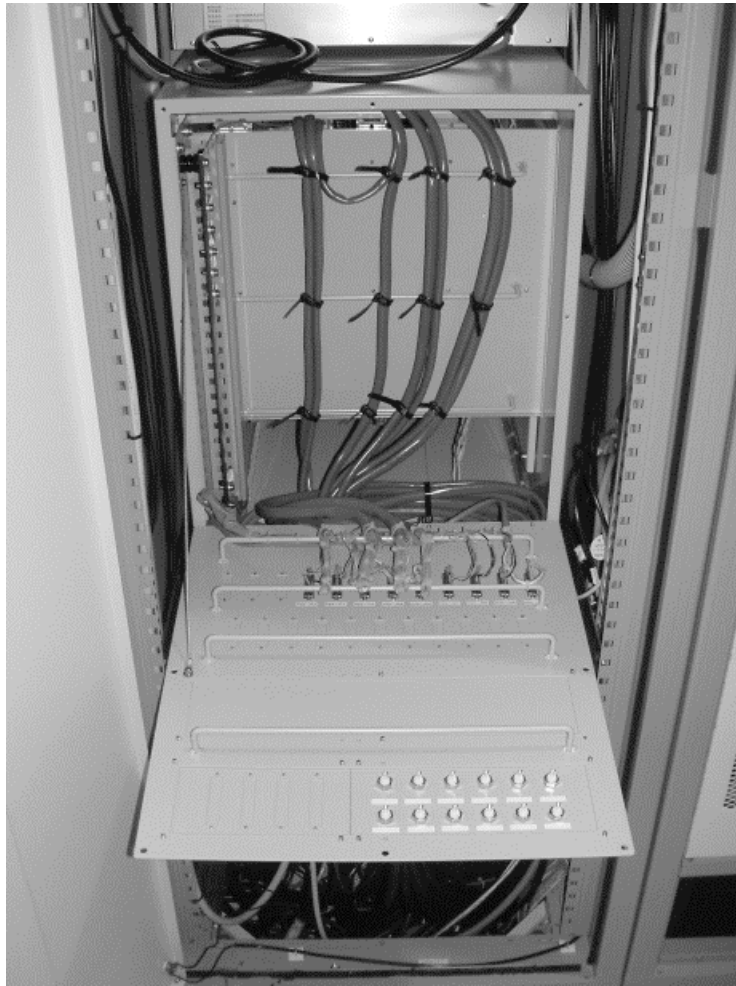
Fig. 3.22. The inside of the rear panel of the new connector box. There are seven bars to tie signal cables.
