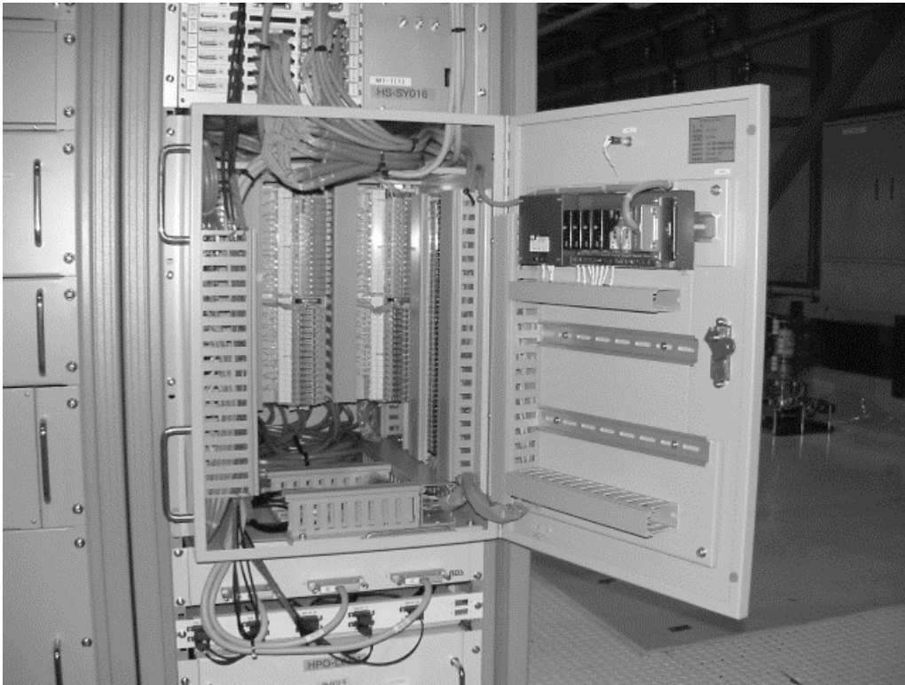
Fig. 3.21. The inside and back of the front door of the new connector-box. There are three kinds of terminals in the picture. A normal terminal for analog signals of the magnet power supplies is settled on the side-wall. A terminal of the back of the front door is an isolation-base terminal for analog signals except for magnet power supplies and WGMs. Four terminals on the inner wall are relay terminals for DI and DO signals except for the magnet power supplies.
